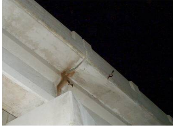
Photo 7: Staining on underside of expansion joint from bat use. Note bats in vicinity*
