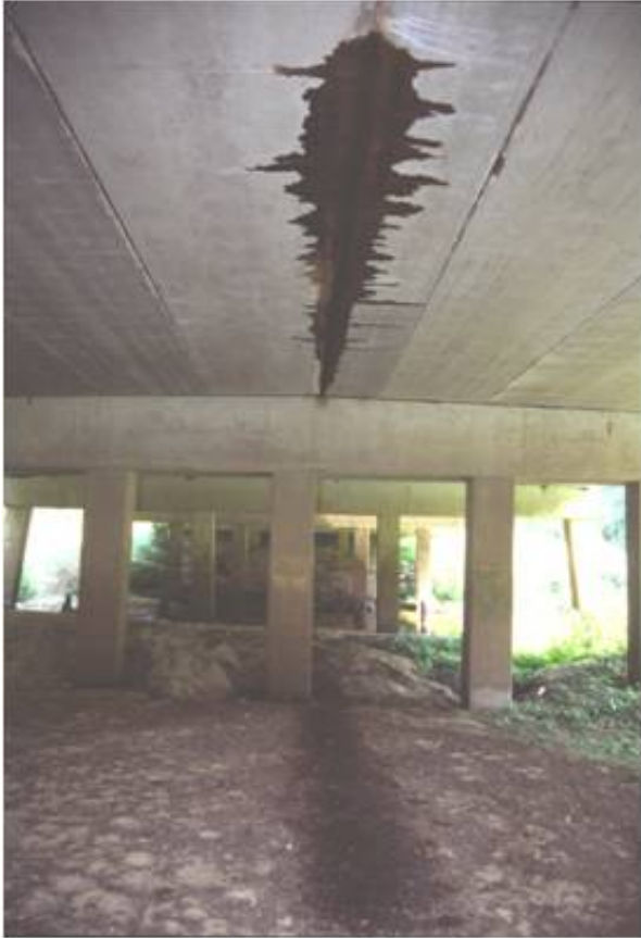
Photo 6: Staining along longitudinal joint. Note guano deposits on ground*
