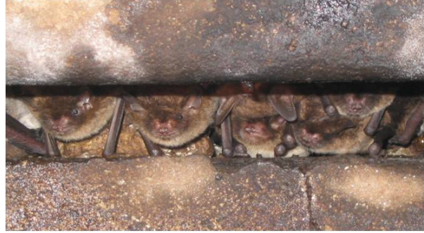
Photo 2: Visible bats within an expansion joint*
