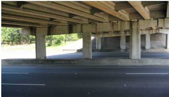
Photo 8: Staining on sides of pier caps*
