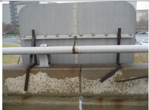
Twisted anchor clamp over the parapet
