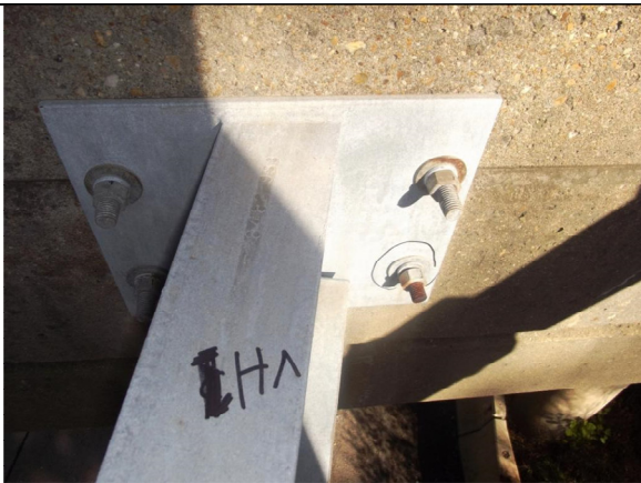
Failed mounting bolt (circled)
