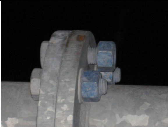
Loose Bolt at splice plate.
