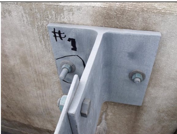
Failed bolt (circled) at parapet mount.
