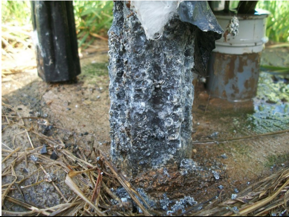
Corrosion with 1/8" deep pitting on breakaway couplers
