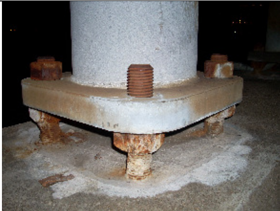
Rusted anchor bolts and missing nut
