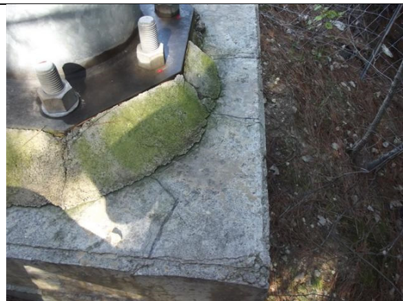
Deteriorated and cracked grout
