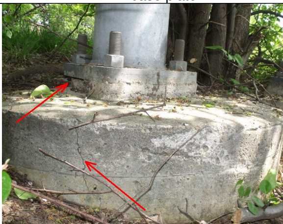
Deteriorated grout pad and cracked pedestal
