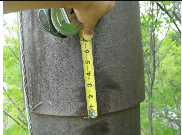
4" vertical crack at the slip joint
