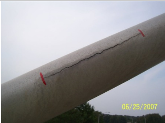
6" crack in lower chord of luminaire
