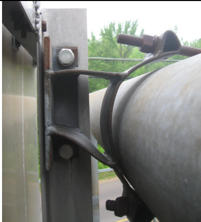
1 1/2" gap between upper chord and connection strap
