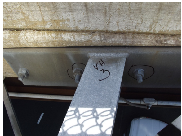
Two failed bolts (circled) at parapet mount
