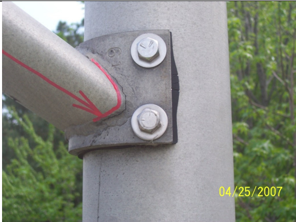
Lower arm of luminaire chord has a 3.5" fatigue crack in weld at connection to pole
