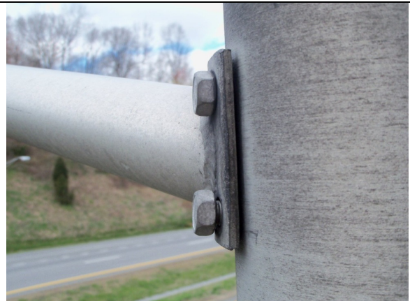
Two of four bolts loose in top chord connection to luminaire pole
