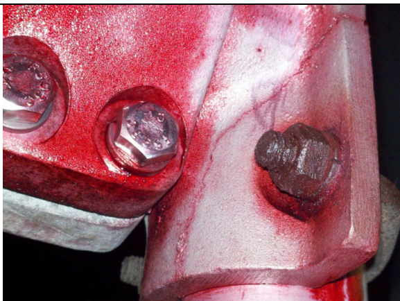
Crack in orbital bracket of 2nd signal from right pole
