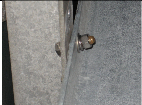
Poor vertical hanger connection with the Z-bar
