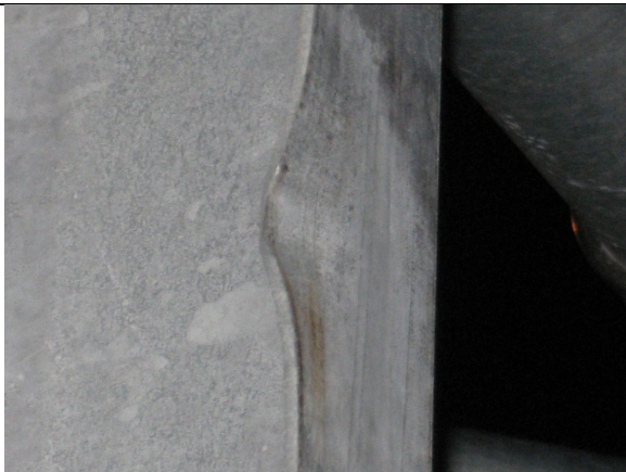
Damaged & bent flange of vertical hanger
