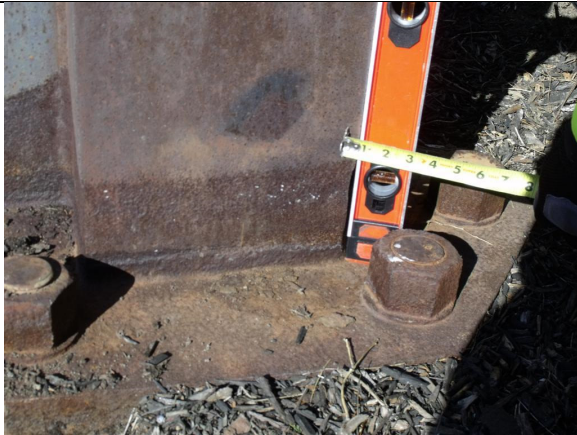
Section loss to the bottom of the pole.
