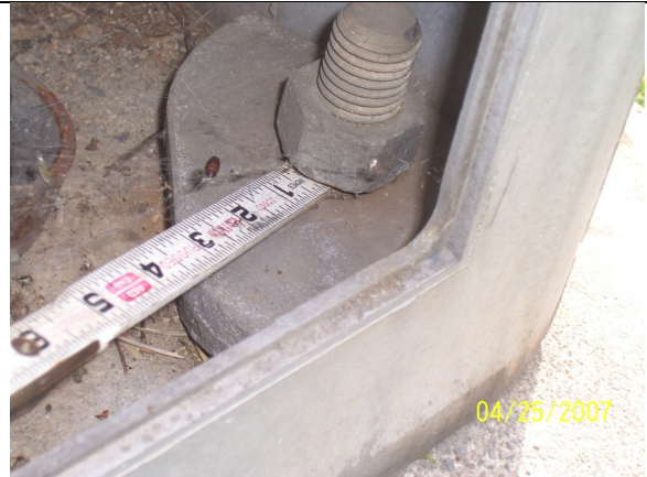
Loose anchor bolt nut at luminaire base
