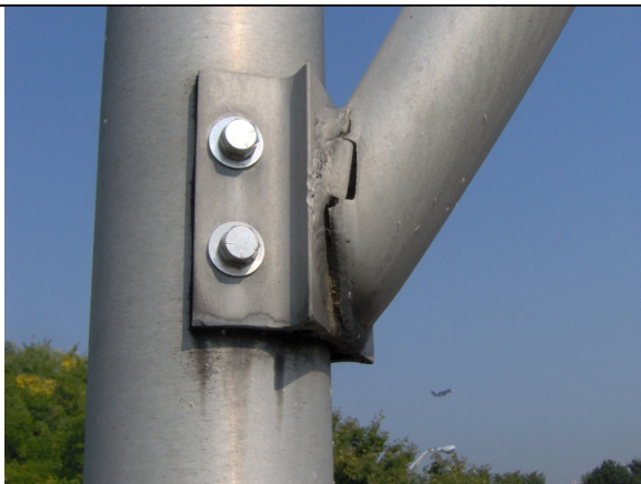
Fracture in weld of lower arm tube to luminaire pole connection
